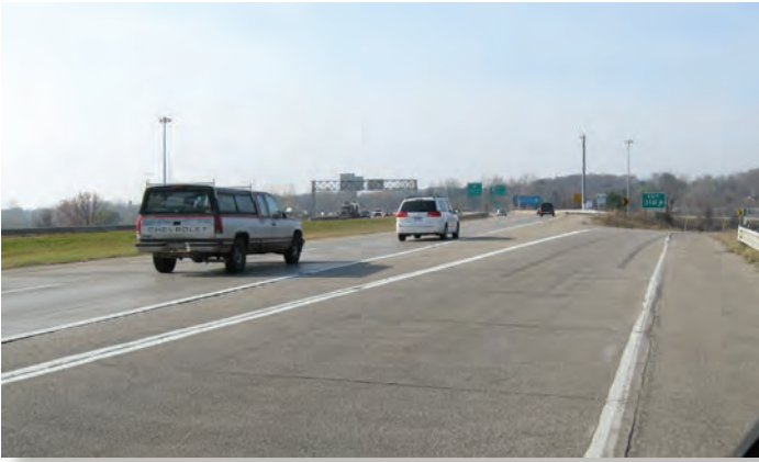
HFSTs can be installed on different surfaces, including jointed pavements when proper masking is used (Image: Michigan DOT)
