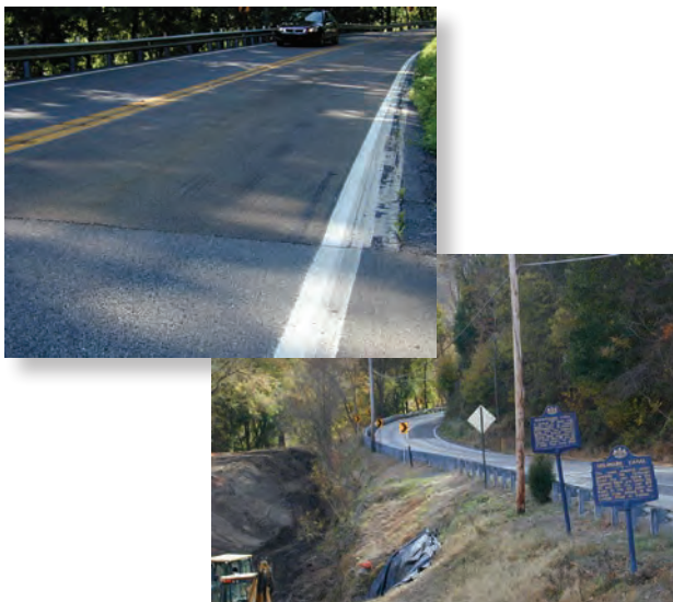
Installation of HFST on SR 611 southbound lane and overall view of the site and its limited right of way (Images: Pennsylvania DOT)
